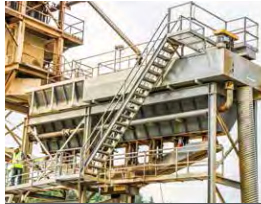
CLASSIFYING TANK WITH STAIRWAY
