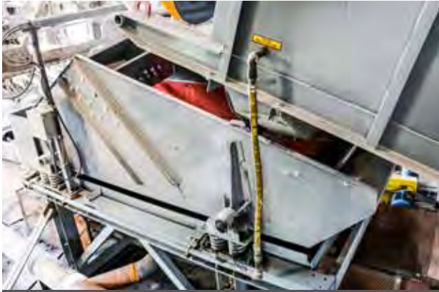
RECYCLE WATER LINE
