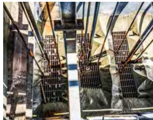
VALVE AND GRATE
