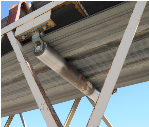
BEFORE: BELT/BACKET DAMAGE
