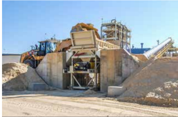
SKID-MOUNTED FEED HOPPER
