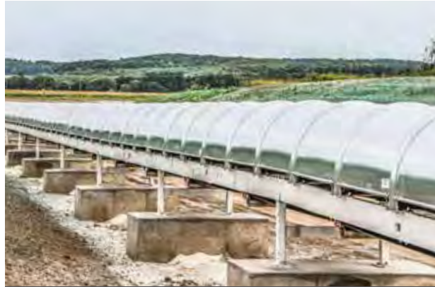
CHANNEL FRAME CONVEYOR
